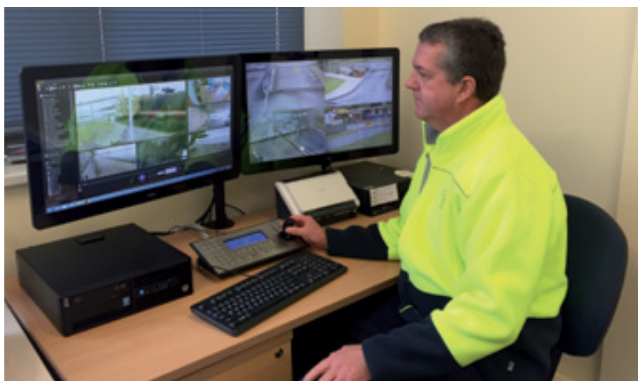
Port of Albany – CCTV monitoring in operation
